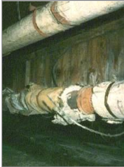
Asbestos insulated pipe in utility space
