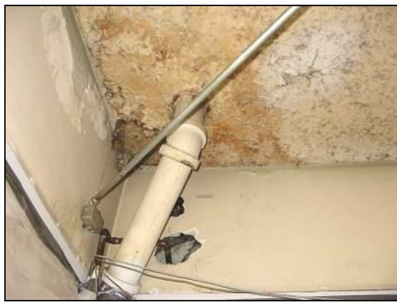
Water damage, deterioration
